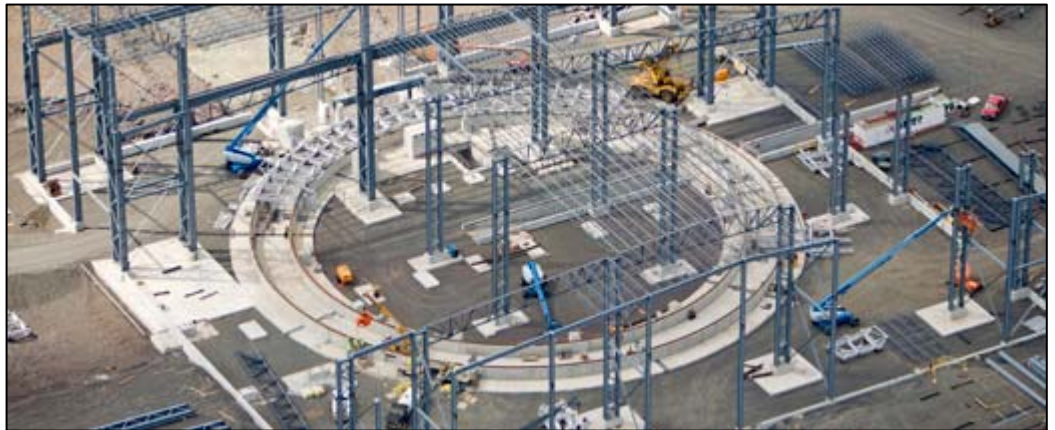
The rotary hearth furnace under construction at the Steel Dynamics ITmk3® plant
